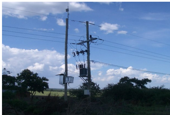
Figure 1 the network node in Nata village. From the top of the left pole, you see a lightning protection rod, a Wi-Fi antenna, a box for the Ethernet switch and the Wi-Fi access point, and another box for back-up power (UPS). The fiber from the right pole comes into the Ethernet switch.
